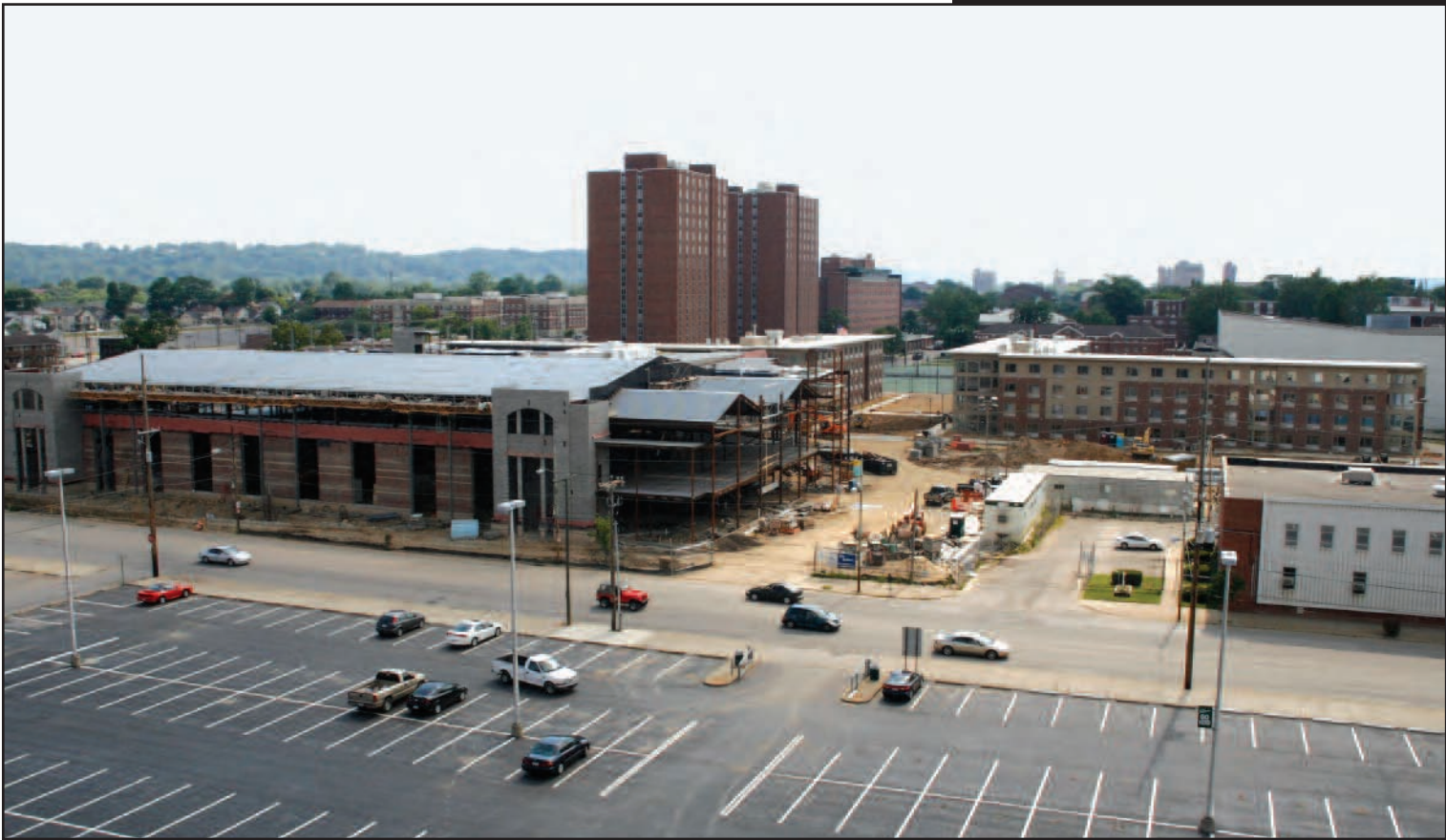
A bird's-eye view of the massive three-story student recreation center (left) which will be adjacent to two new First-Year residence halls (right). University officials hope these state-of-the-art facilities will entice more incoming students to live on campus.
