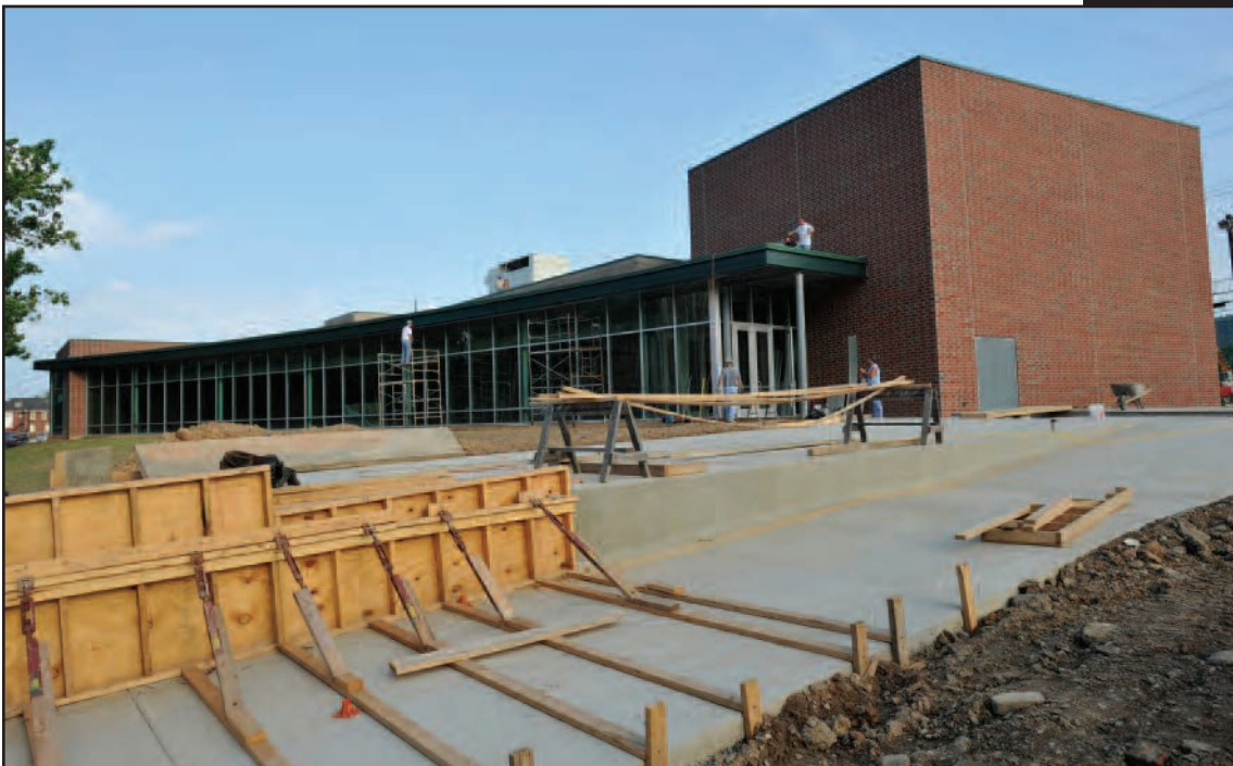
The new lab facility for the College of Information Technology & Engineering is nearing completion.
