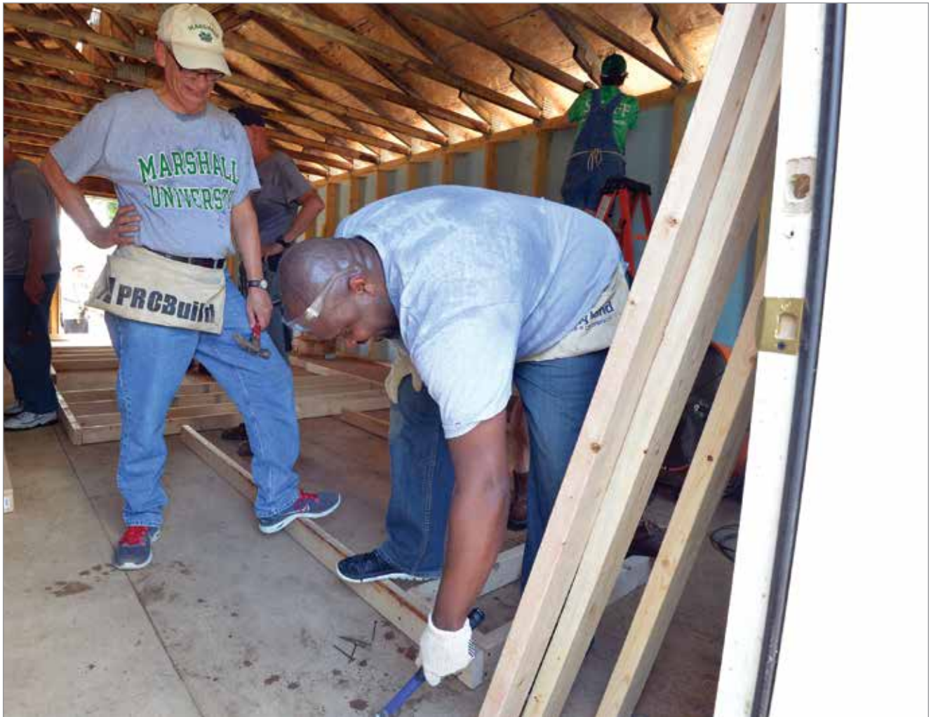
Marshall President Jerome Gilbert and Cedric Gathings joined other senior administrators from the university to help with a Habitat for Humanity project in Huntington on July 15, 2016.
