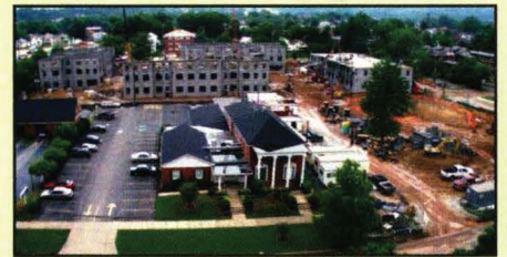
The Erickson Alumni Center sits amid the current construction site of a new student housing complex.
