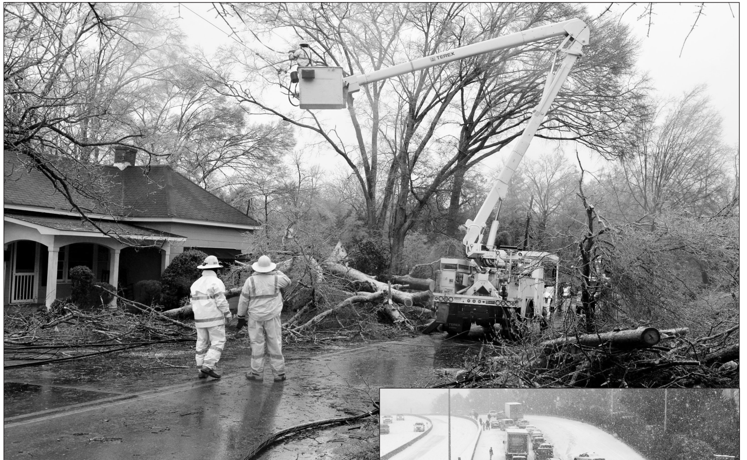
KENT D. JOHNSON | ATLANTA JOURNAL-CONSTITUTION | MCT ABOVE: Griffin Power employees work on downed power lines during the winter storm on Maple Drive in Griffin, Ga., Wednesday.
