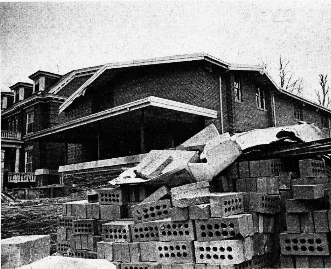
SIGMA ALPHA EPSILON HOUSE RISES AT 14TH STREET, FIFTH AVENUE ... Will house 42 men, have ballroom
