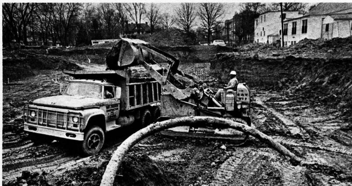
WORKERS FROM Ray and Tassen Construction, Inc. are in the process of removing 28,000 cubic yards of earth during the construction of the new student center. Completion date set for August, 1970.
