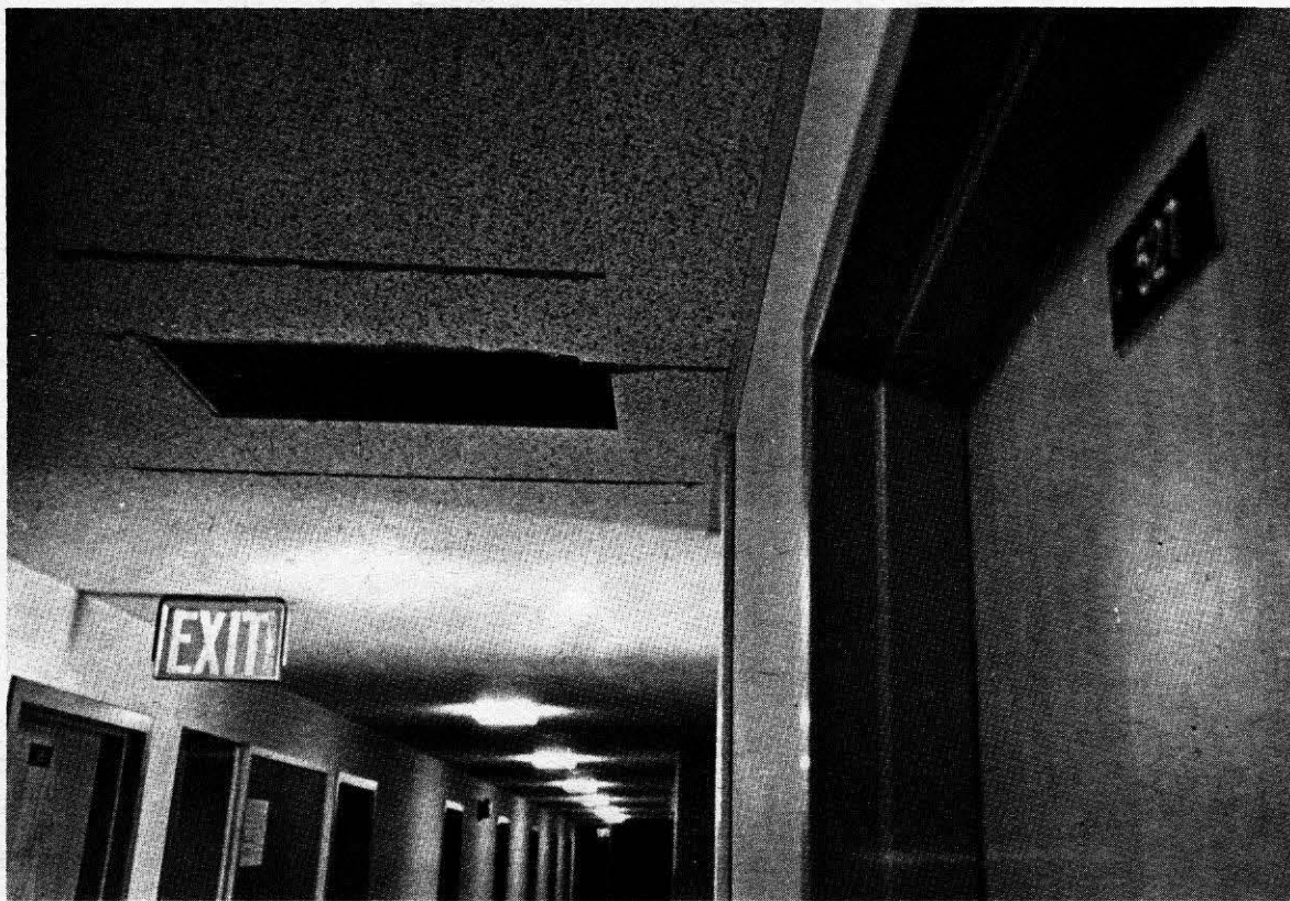
PART OF CEILING KNOCKED OUT IN SOUTH HALL ... one of the most common forms of damage
