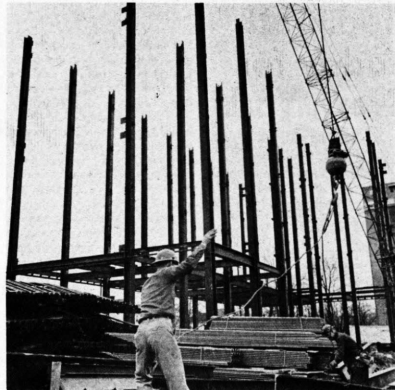
THE GIRDEERS FOR the twin towers rise from their foundations which the Kroger warehouse occupied. When finished, the 17-story twin towers, housing both men and women separately, will be the highest building in Huntington.
