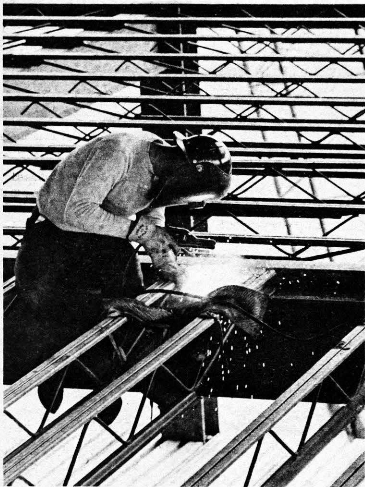
THIS WELDER is in a "web" of steel as he connects steel floor supports to a main beam on an upper floor of the Twin Towers project.
