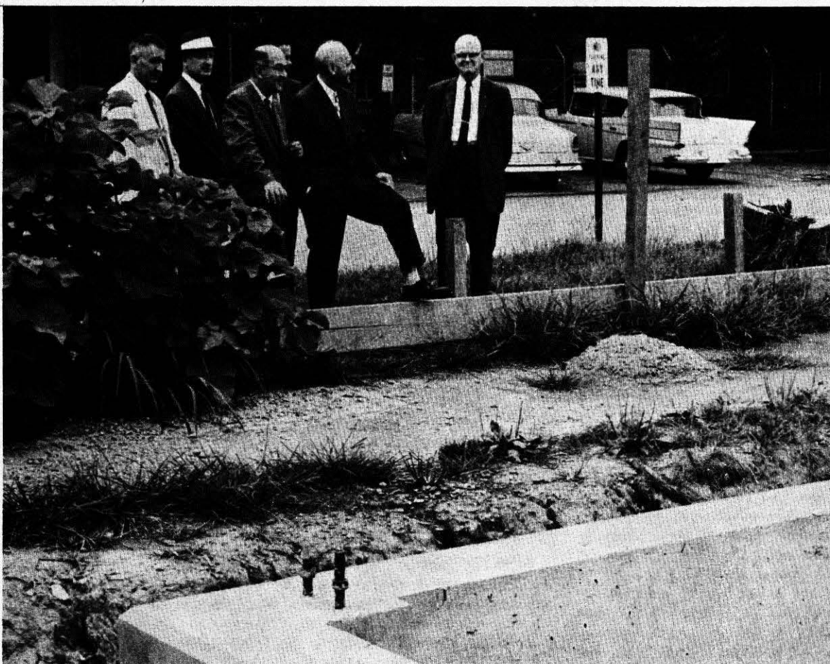
Members of the West Virginia State Legislature's interim sub-committee on higher education examine the building progress on the new physical education building. President Stewart H. Smith conducted the legislators on a tour of the campus during their visit Monday.
