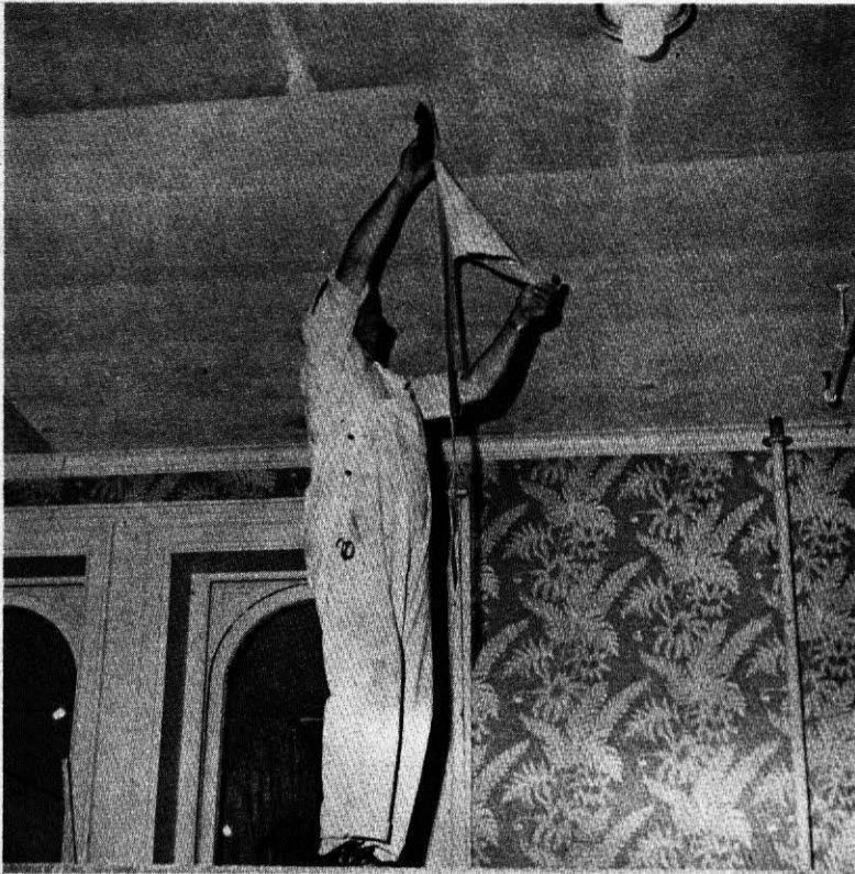
North Parlor of Old Main, which is used for college receptions, has been undergoing repairs and redecoration during the past week. The woodwork is to be painted and the ceiling repainted.
