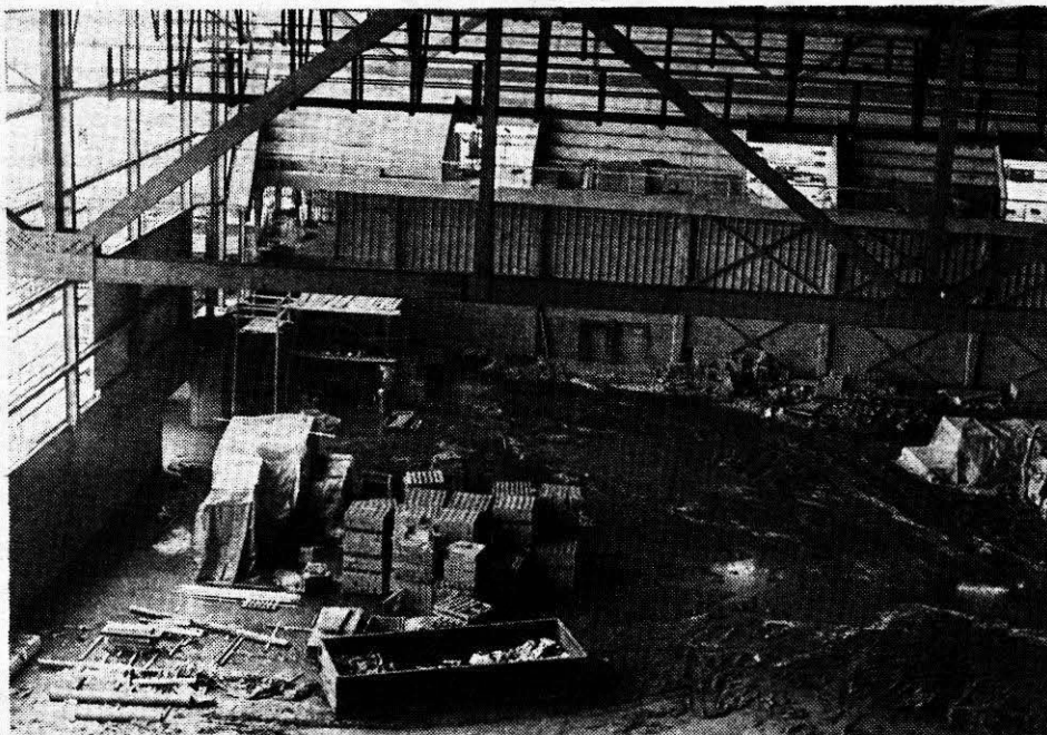
Beams, girders and pipes, symmetrically patterned, rise majestically above cinder blocks, tractor marks, and other construction paraphernalia of what will be the future "Herd Heaven —" Cam Henderson Center. --Photo by Bradd Smith.
