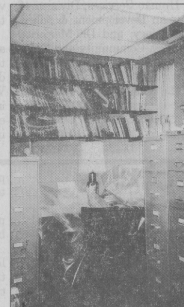
photo by Nicole R. Pickens Dr. Charles O. Lloyd keeps plastic over his books and desk to protect them from Harris Hall's leaky roof.
