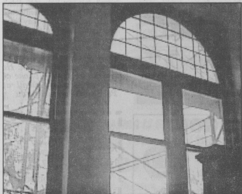
The windows in the main stairway of Old Main usually allow students and faculty to look out onto the campus. Now the view is marred by scaffolding while the brick is being cleaned.
