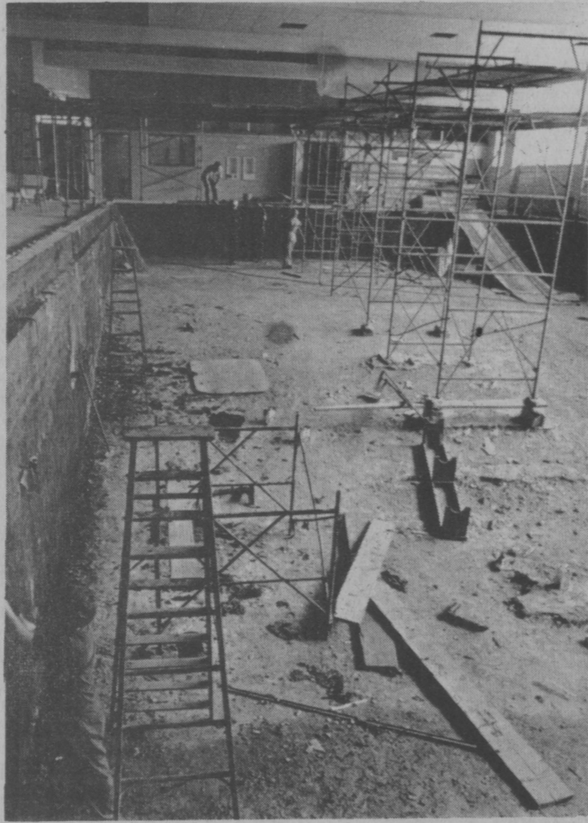
WORK ON POOL CONTINUES Due to be finished in September (Photo by Lew Harford)
