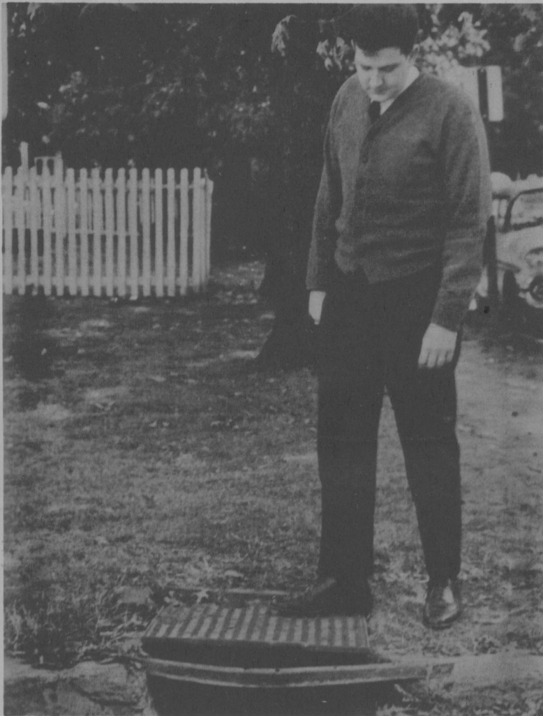
EDITOR-IN-CHIEF LARRY ASCOUGH ... Views Crumbling Storm Drain
