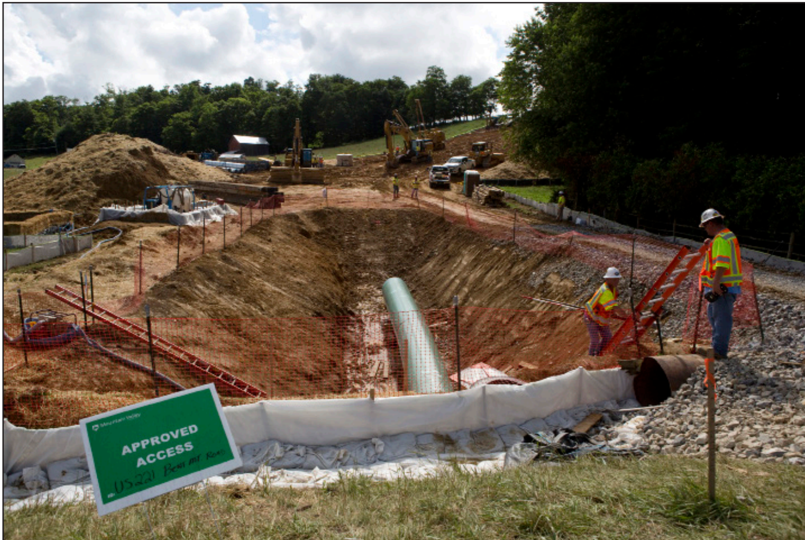
Construction of the Mountain Valley Pipeline, which will run through Virginia and West Virginia.
