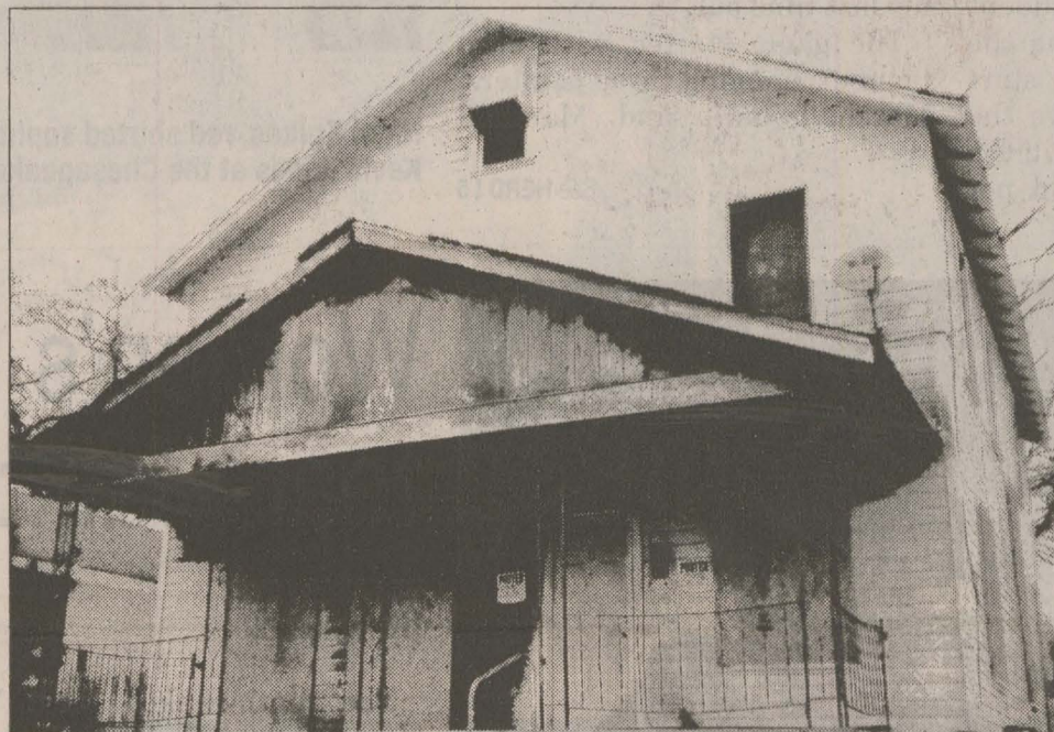
The City of Huntington is working to beautify the city by demolishing houses and structures that have fallen into a state of disrepair.
